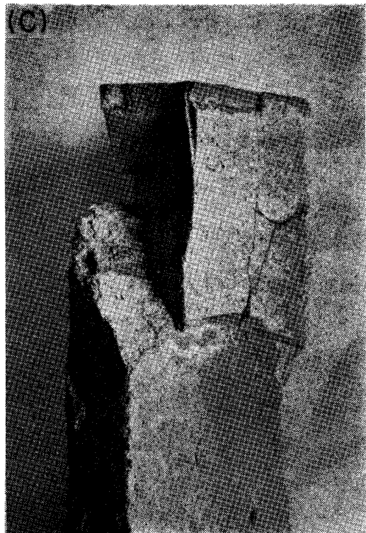
(a) Size (b) Arrangement (c) Crack of hatched region Photo. 3. Cracks of fire clay bricks.
