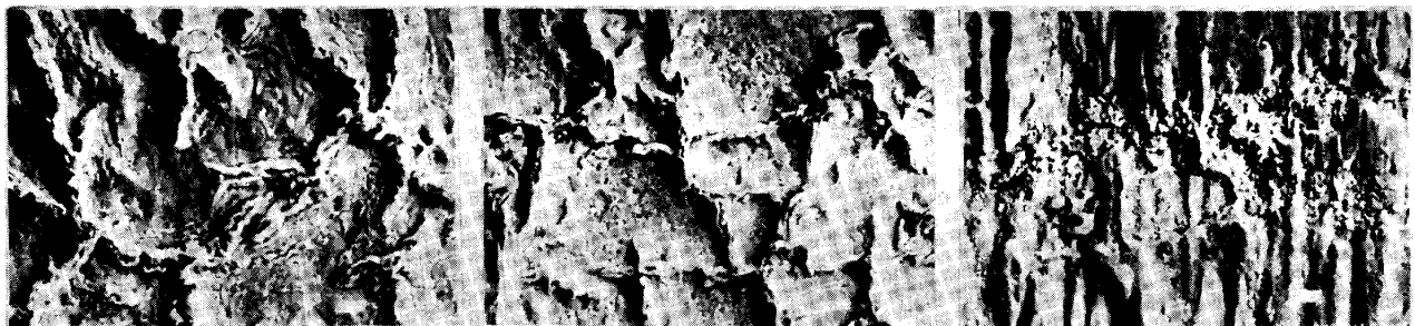
b) Mechanical and thermal stress c) Thermal stress d) Air cooling thermal stress
